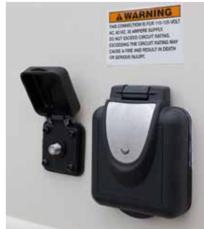
Typical park-supplied cable TV hook-up located on the left side of the motorhome
