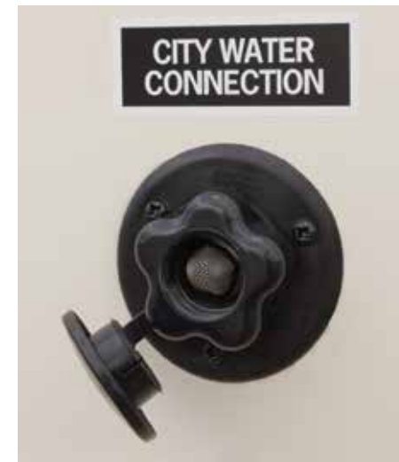
Typical city water fill
