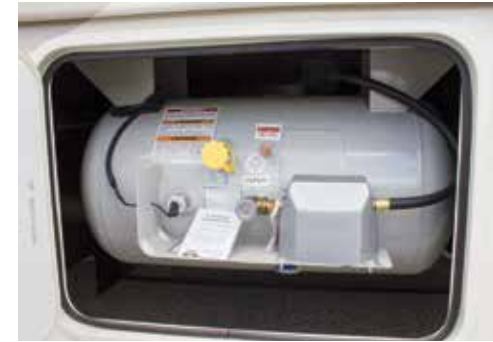
Typical propane gas tank
