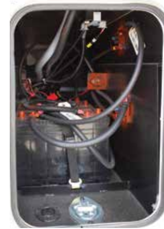
Typical Class A motorhome auxiliary battery compartment
